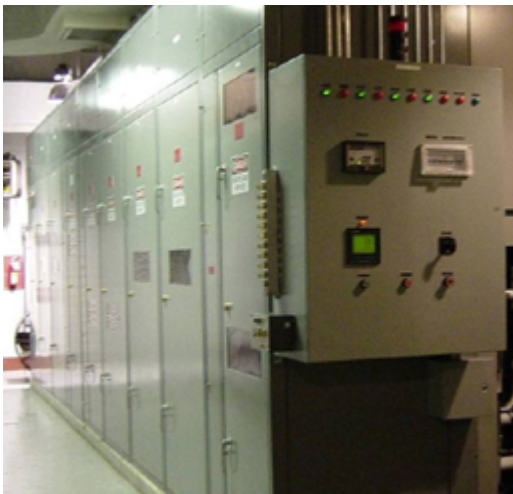
MV Equalizer system in a hospital, USA
