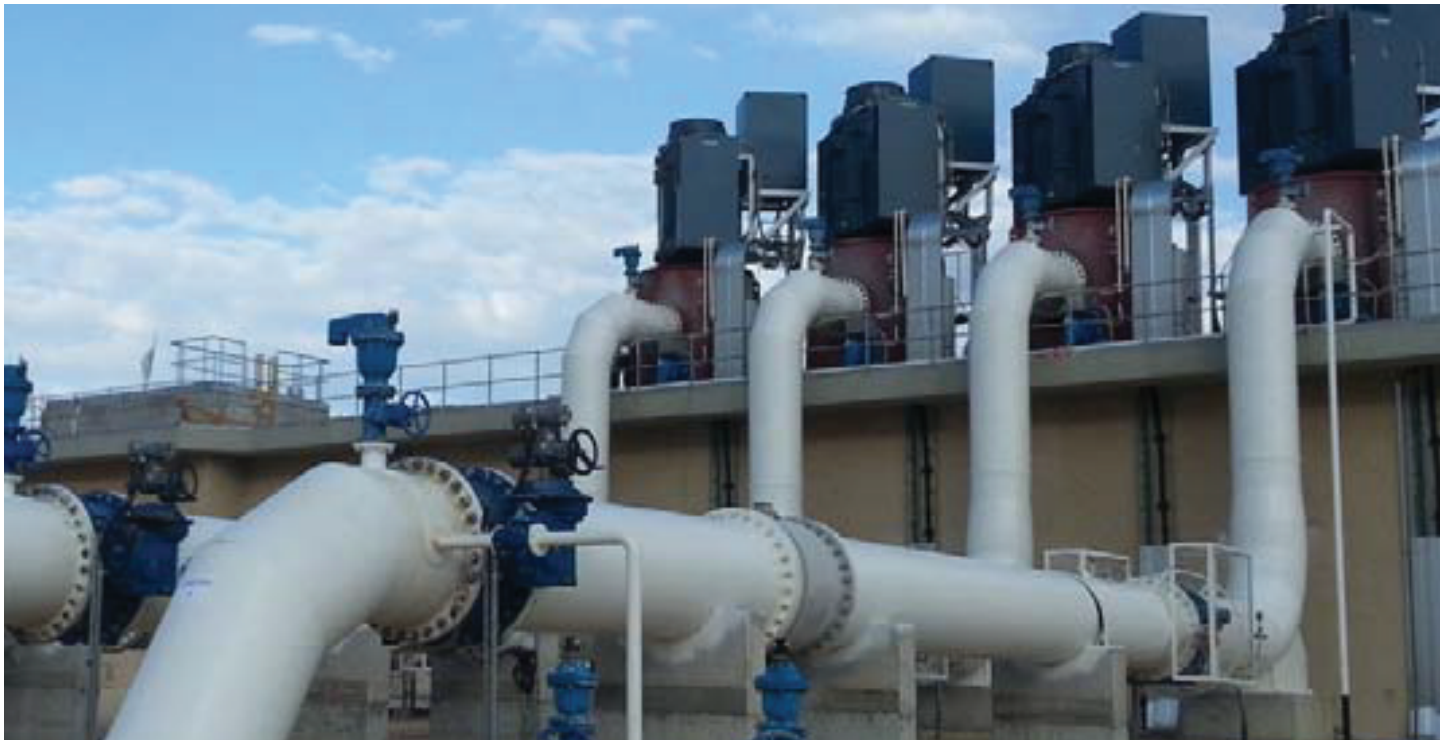
Water pump station at Mekorot Israel
